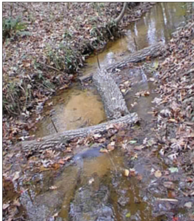
Figure 4. Artificial debris dam installed as part of a pilot-scale stream restoration project, sponsored by the US Department of Defense, Strategic Environmental Research and Development Program, at Fort Benning, GA. Restoration that promotes the storage of organic matter through the creation of debris dams has the potential to decrease downstream N loading.
